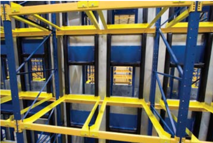
Seals are created at the back of each pallet location, forcing the air to travel through the pallet of product, resulting in better airflow, which leads to more efficient freezing.
